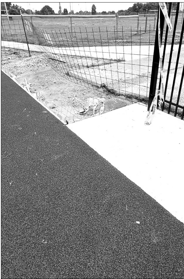
While not necessarily visible in the photo, footprints were left behind permanently damaging the PIP surface.
