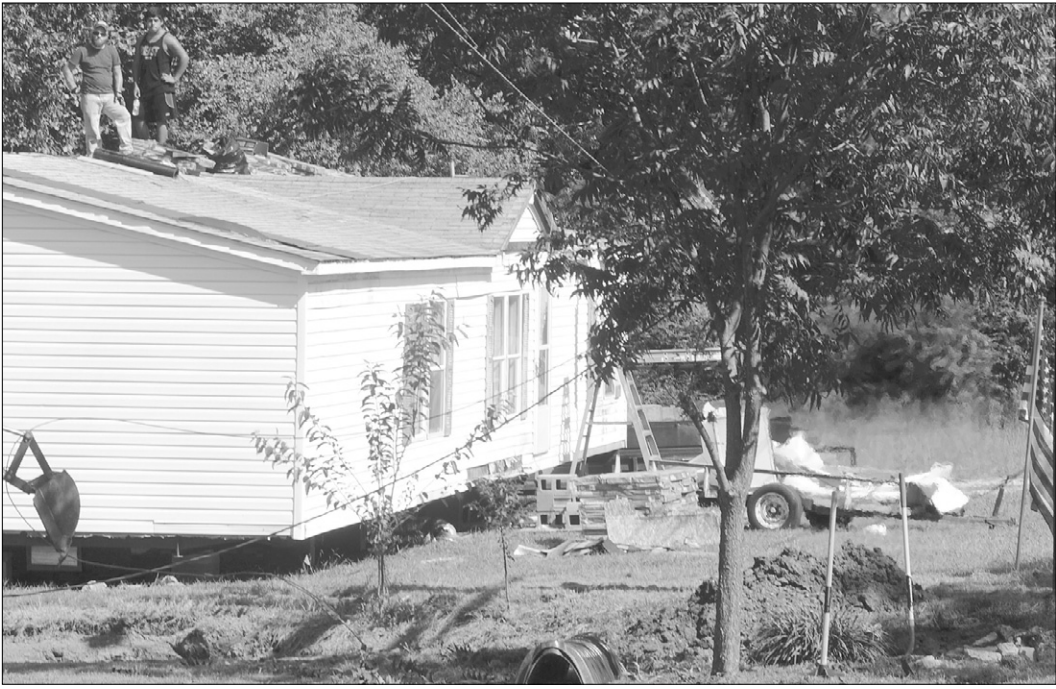
Two digging shovels mark the spot where a natural gas fire erupted from a ruptured natural gas line.
