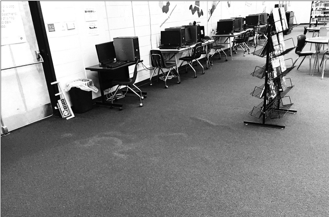
Rain-soaked carpet in the MMS Library.
