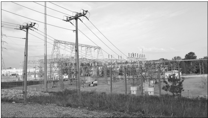
New high-wattage breaker located near the Noranda plant in Huntingdon. Photo by Joel Washburn
