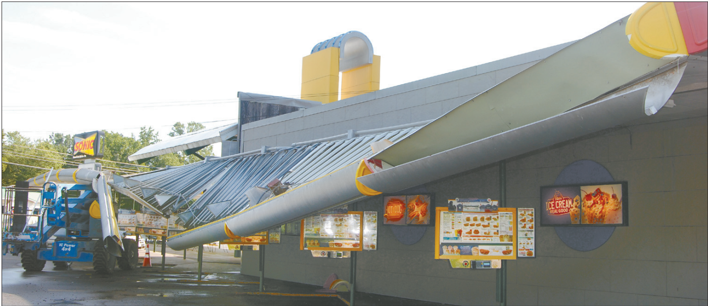
Above, Torrential rainfall is suspected of collapsing an awning at Sonic Drive-In in Huntingdon. Below, The home of Richard and Carolyn Brooks was heavily-damaged by the storm. Photos by Ernie Smothers/The Banner
