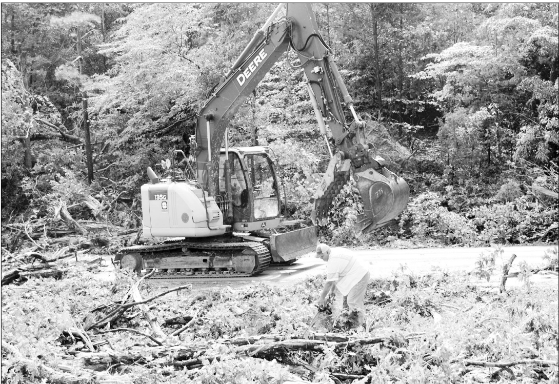
Top, A large spruce tree rests on Mrs. A.P. Fry's home. Above, TDOT employees utilize a trackhoe and chainsaws to clear storm debris from a section of Highway 70 in Cedar Grove. Photos by Ernie Smothers/The Banner
