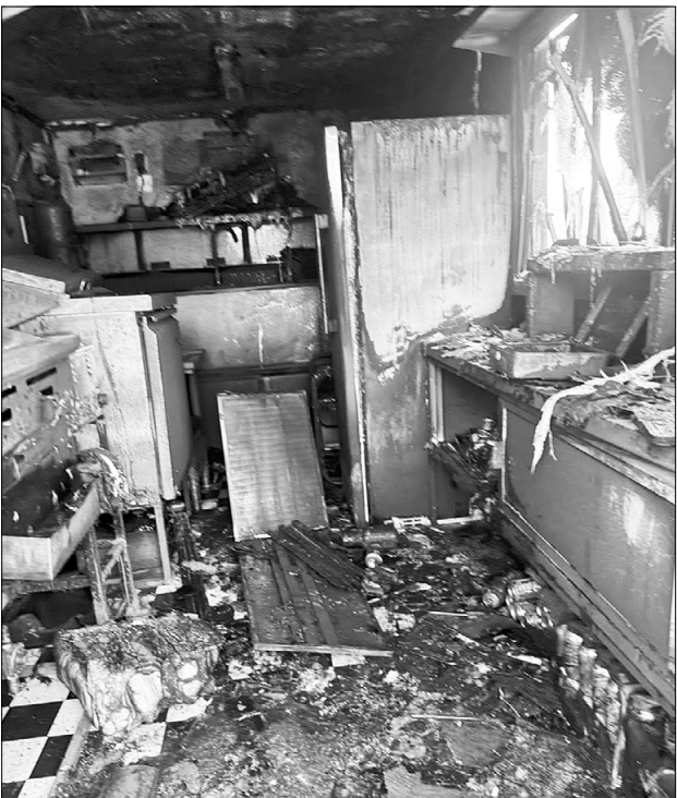
The interior of the TNT Tacos truck following Thursday’s explosion. Submitted photo
