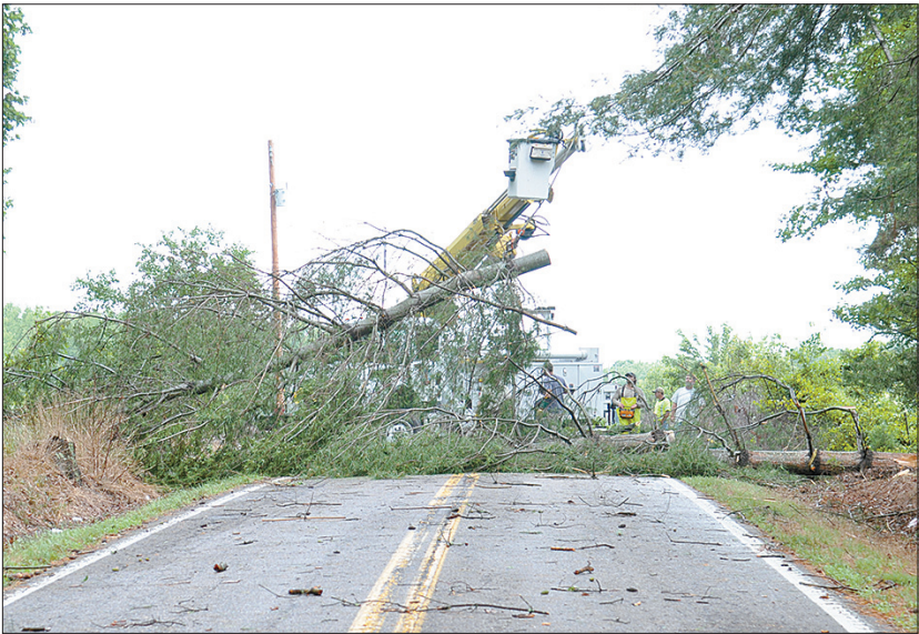
CARROLL COUNTY (June 1) — The Carroll County Electric Department and the Carroll County Highway Department responded to scenes of downed trees blocking roads near Christmasville in western Carroll County Monday morning following a brief but intense storm. Trees and utility lines were down on TN-190 (pictured), and very nearby, a large tree partially blocked Hinkledale Road. Photo by Brad Sam/The Banner
