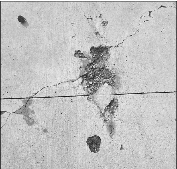
The concrete surface at the Carroll County Inclusion Park is chipped in many areas. A closer view of one chipped spot shows the extent of the damage. Photo Courtesy of Carroll County Inclusion Park
